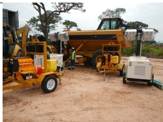
New pumping and lighting and equipment
