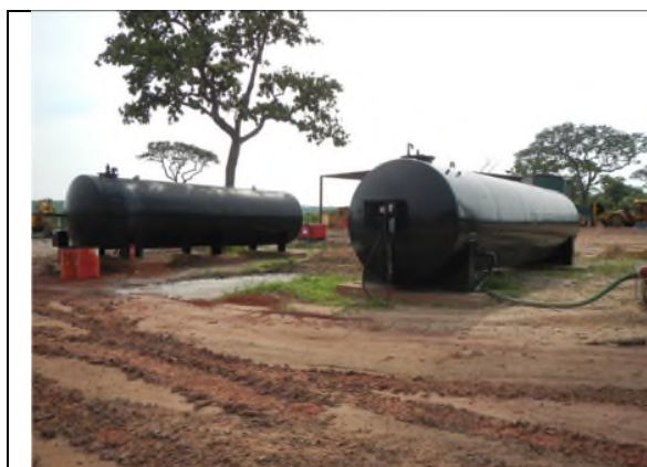
Infrastructure - diesel storage
